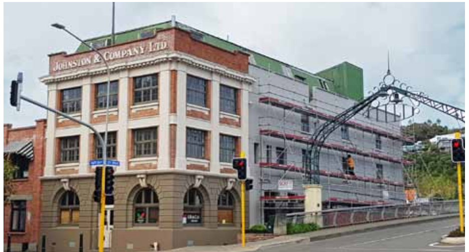
Johnston & Co, winner of Whanganui's 2023 supreme heritage award, is now strengthened and fully restored.
