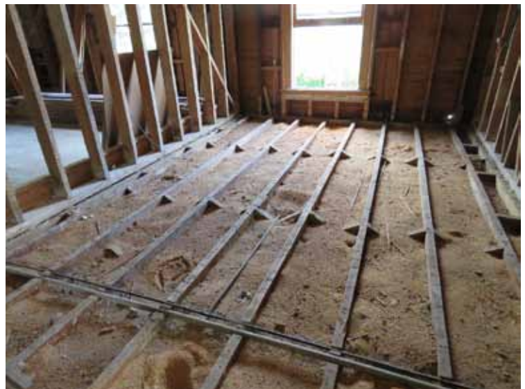
First floor, flooring removed. Showing sawdust and pumice sound deadening, gas pipe for lighting, tops of herringbone struts between the floor joists. Ann Galloway
