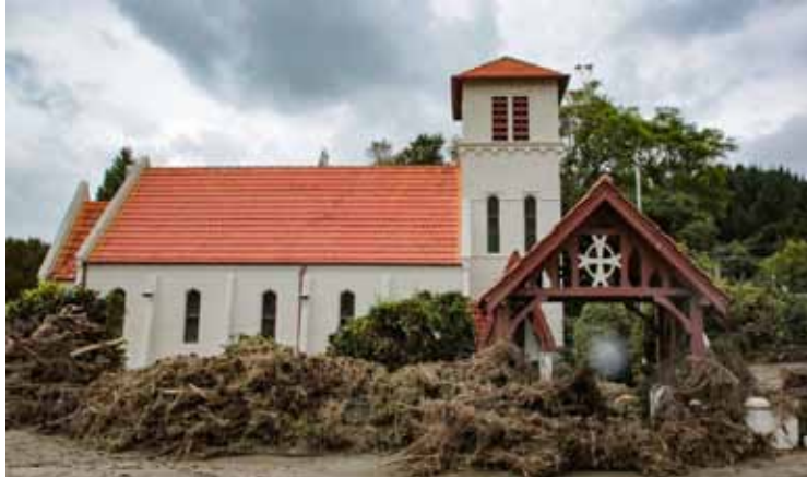
Eskdale War Memorial Church surrounded by silt and slash. Source: Hawke's Bay Today 18 February 2023
