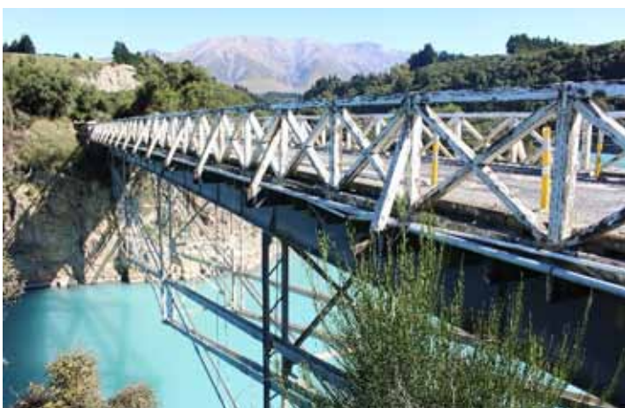
The damaged balustrade prior to repair.
