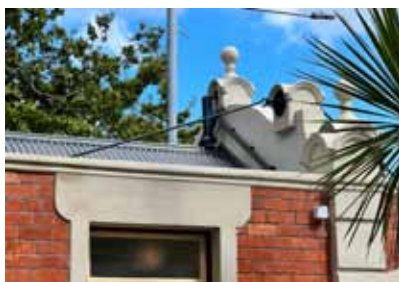
Discrete steel framework to back of strengthened parapet after completion of the works
