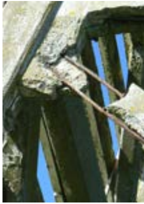
Concrete disintegrating under pressure from expanding corroding steel.
