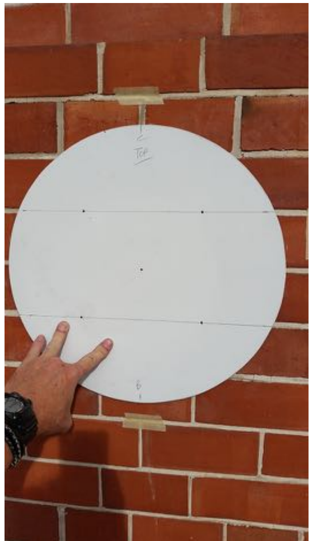
2) Position aluminium (ACM) backing plate and mark out hole locations for screw fixings - to align with mortar joints
