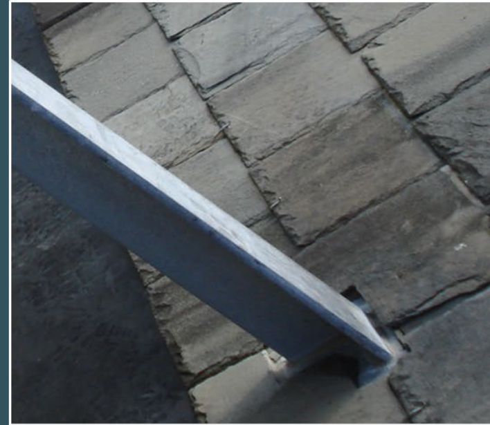
52 penetrations to slate roof reliant on sealant
